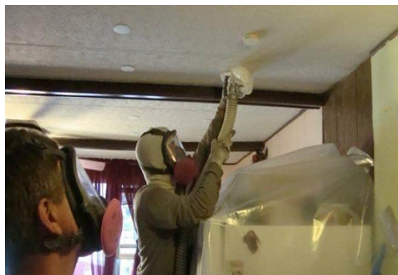
Installing insulation through the ceiling: The technician pushes the fill-tube into the cavity and out near the edge of the roof. The holes are drilled in a straight line for appearance sake.
