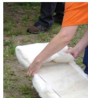
Batt stuffing: When this method works, it is quite efficient. Wall cavities with obstructions or non-standard widths must be blown.
