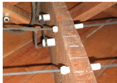
Knob-and-tube wiring: Prior to insulating around knob-and-tube wiring, barriers must be installed to keep insulation at least 3 inches from the wires.
