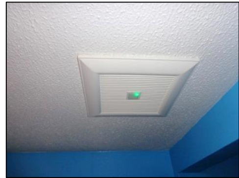
Surface-mounted exhaust fan: Exhaust fans aid air quality by drawing fresh air into the building as they remove indoor pollutants.
