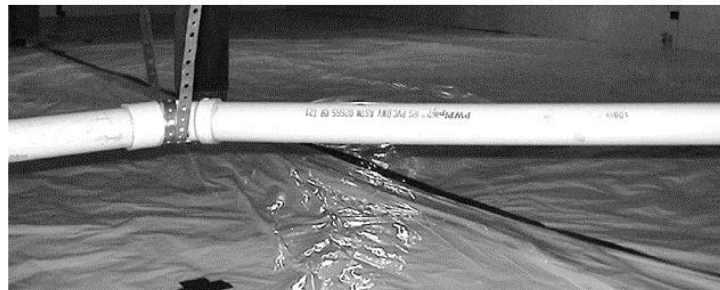
A well-sealed crawl space: The dirt floor in this crawl space is covered with a well-sealed cross-linked polyethylene ground moisture barrier.
