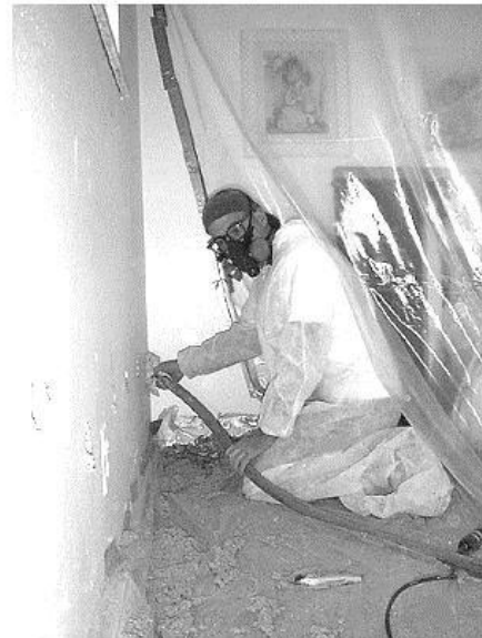
Wall-blowing tent: This tent protects the customer and their belongings from insulation and paint dust.
