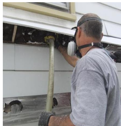
Tube-filling walls: Insulation is dense-packed into walls using a fill tube inserted into the wall cavity.
