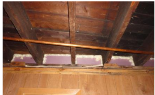
Insulating and air sealing rim joist: Rigid board insulation installed in joist cavities, with spray foam to seal at the edges.
